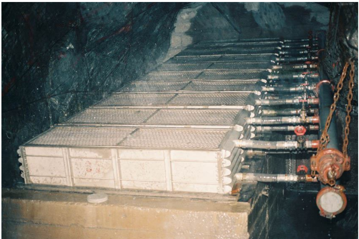
An Underground Bulk Air Cooler with a capacity of 1 750 kW
